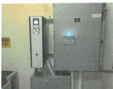
SBR Blower Control Panel
