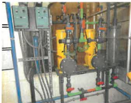
Polymer Storage and Pumps
