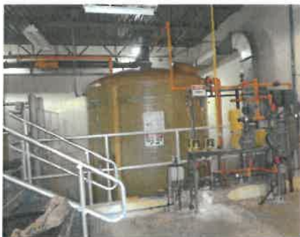
Caustic Storage Tank
