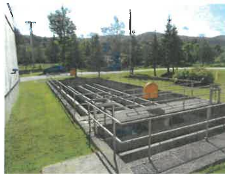
Chlorine Contact Chamber
