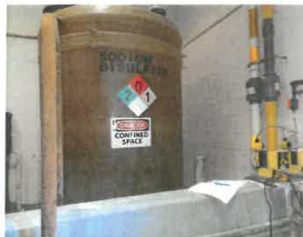
Sodium Bisulfite Tank and Pumps
