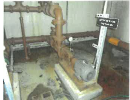
Centrifuge Sludge Feed Pump
