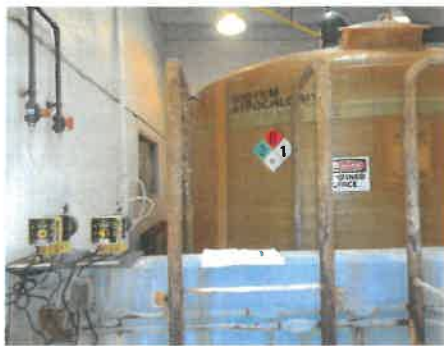
Sodium Hypochlorite Tank and Pumps
