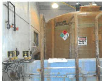
Sodium Hypochlorite Tank
