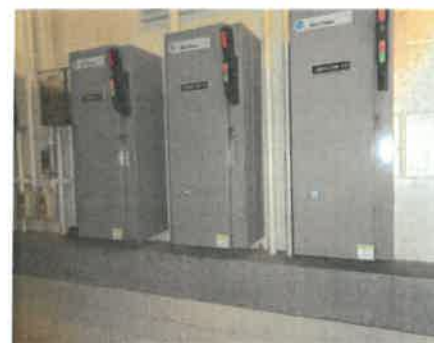
Sludge Conveyor Control Panels
