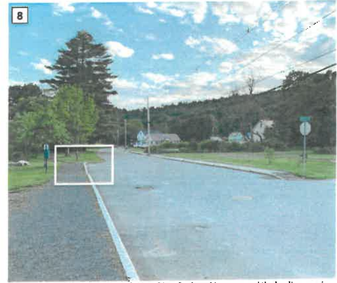
There is only one curb cut next to the Dog River Park parking area, and the landing area is not paved
